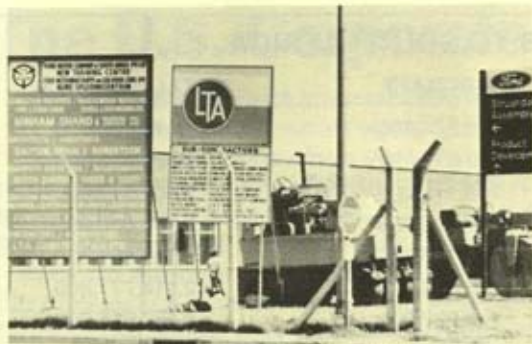
Construction under way at a Ford Motor Company plant in Port Elizabeth, in the strife-torn eastern Cape Province. /Africa News
